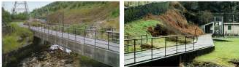
Surface troughing crossing the river Etherow and entering the Woodhead tunnels (carrying six 400kV cables - a double circuit)
